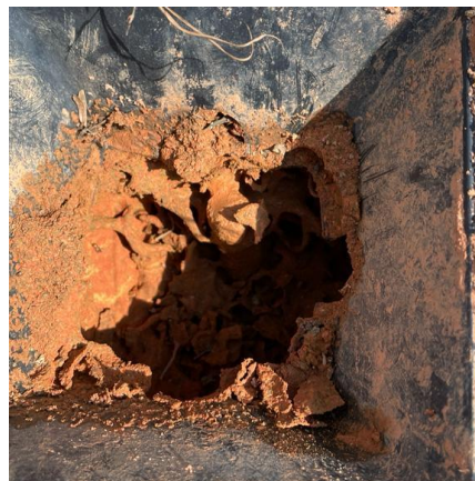
Figure 9. Earthing system with Sodium Chloride on day 72
